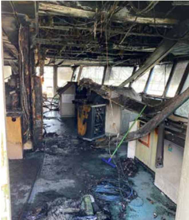
The damage to the bridge. (Source: United States Coast Guard and NTSB marine accident report MIR-23-23)
